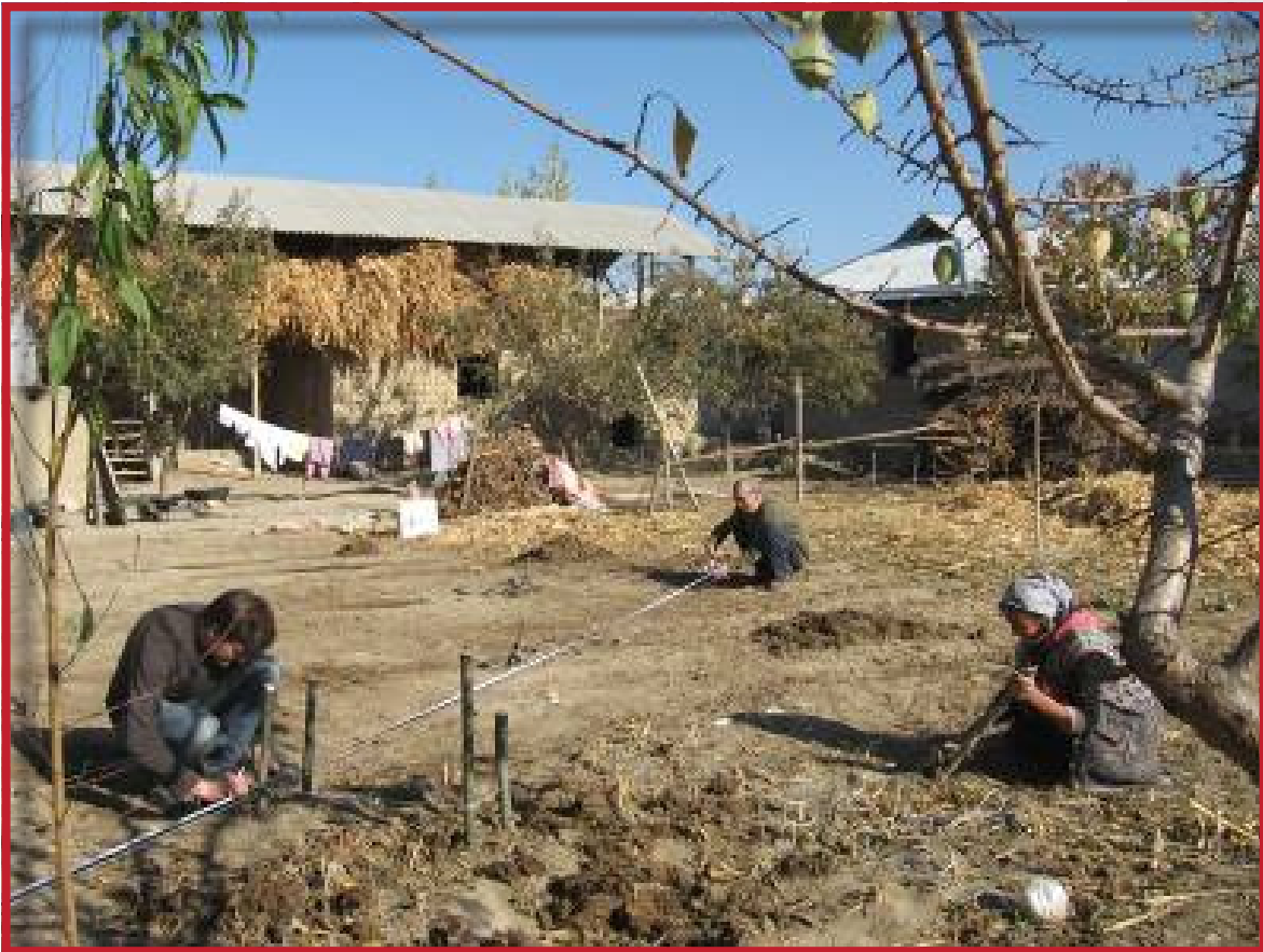
Site markings for greenhouse. Laying out the foundation for additional raising walls.
