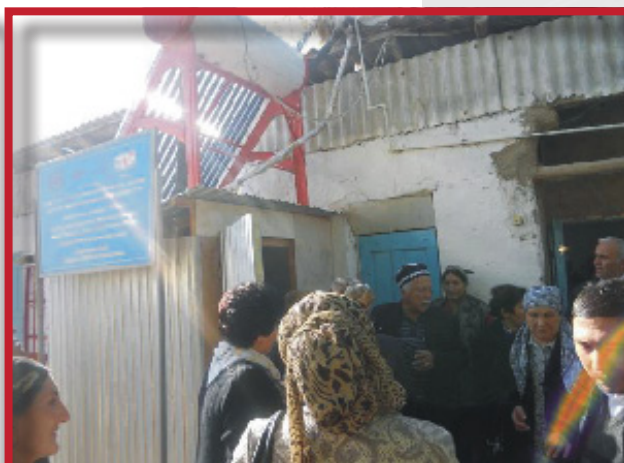
Model – solar collector that provides heating water in the kitchen
